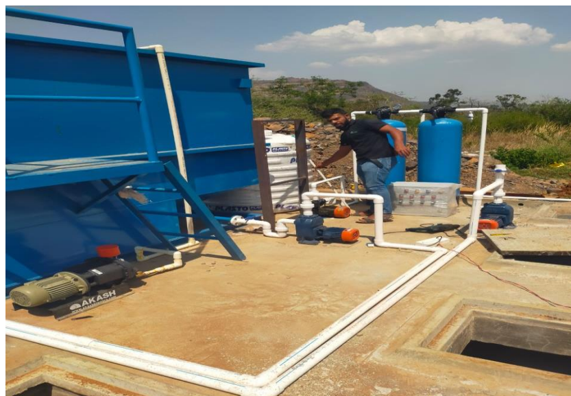
SEWAGE TREATMENT PLANT
